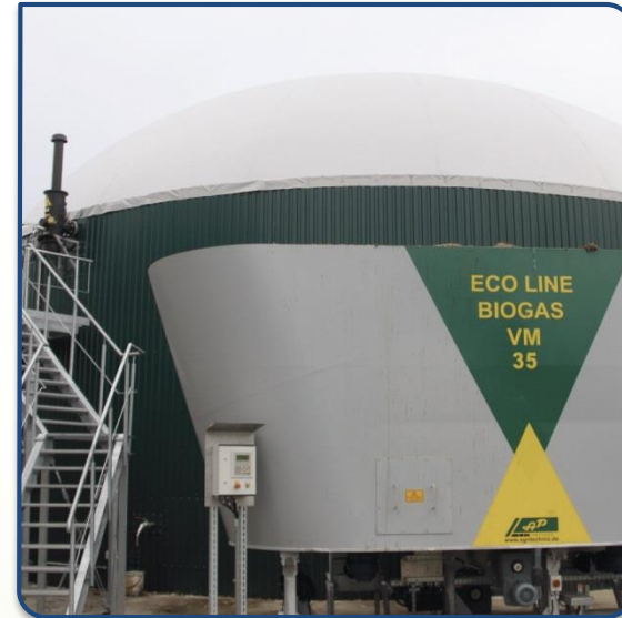
Biogasanlage in Hohenlockstedt
